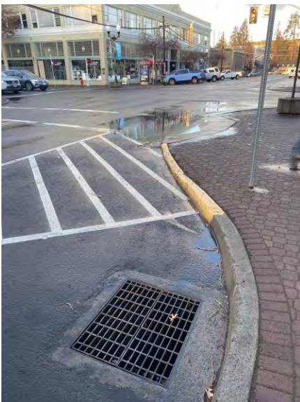
Catch basin next to ponding in crosswalk at NW Oregon & NW Bond
