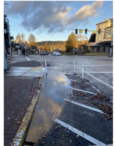
Ponding on road and crosswalk at NW Wall & NW Greenwood
