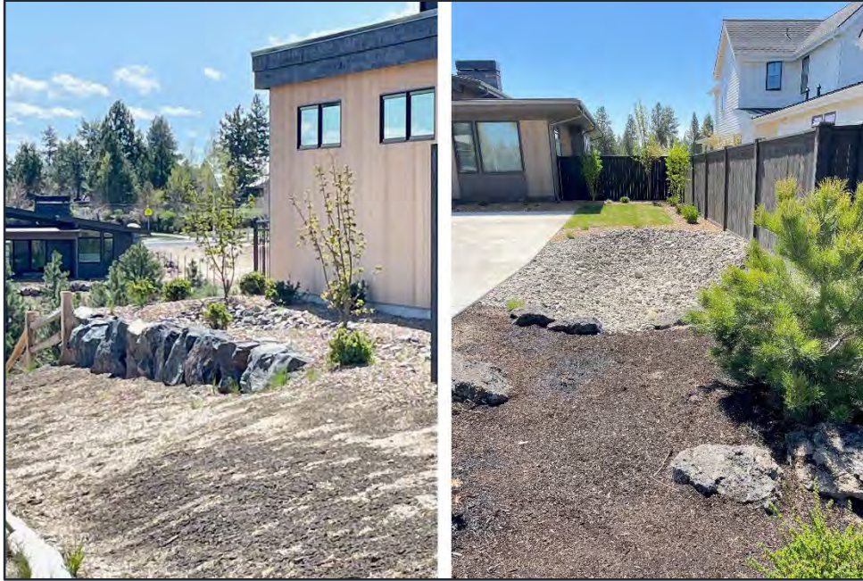
Figure 5. Collage of photographs of stormwater management facilities on lots in Discovery West Ph 5, showing proximity to lot lines, foundations, retaining walls, and steep slopes.
