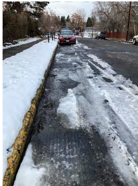
Frozen catch basin on NW Congress St
