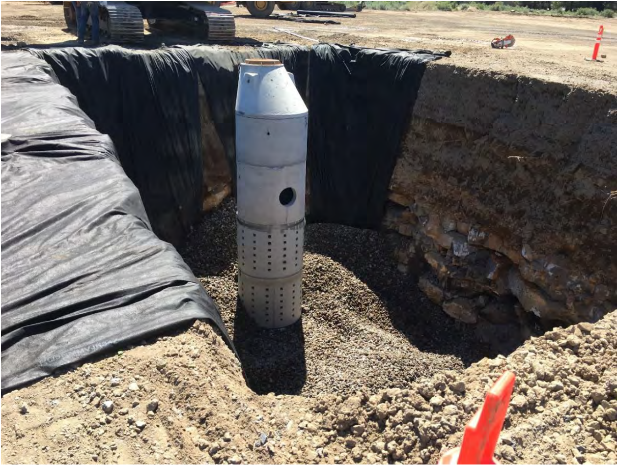
Figure 17. A large drywell installation at Caldera High School.
