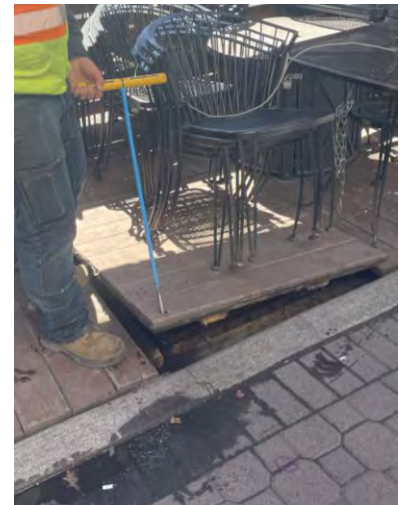
Storm facility access on NW Franklin
