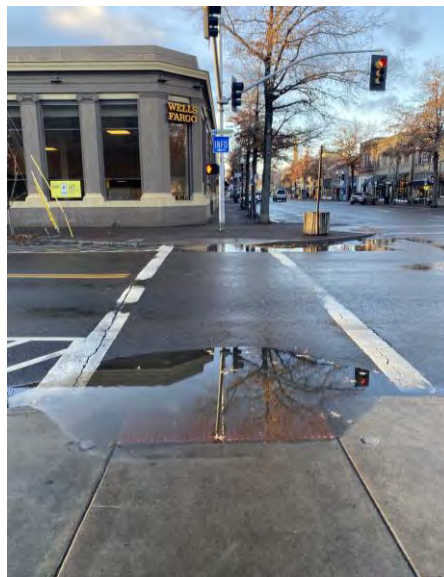
Ponding on ADA Ramp at NW Oregon & NW Wall
