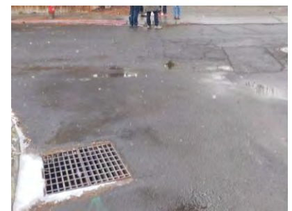
Catch basin at SE corner of NW Riverside and NW Hixon
